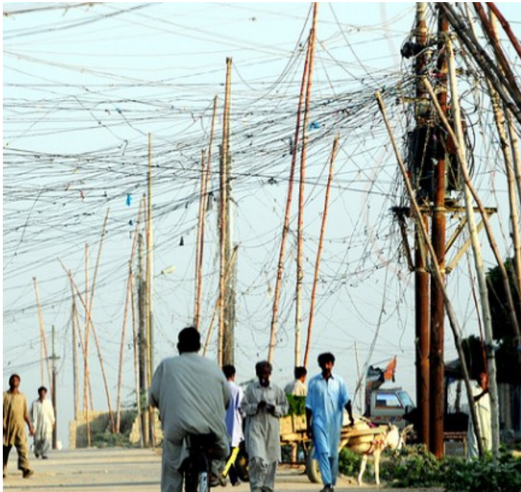
Maze of illegal connections in Pakistan. ( Business recorder )
